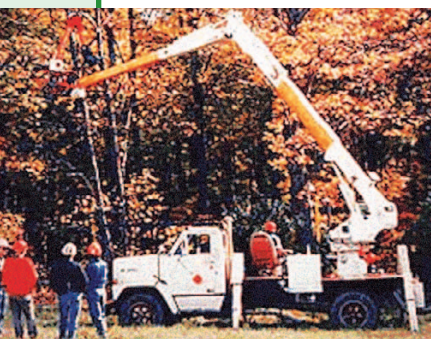
Slave manipulator mounted on the aerial boom
