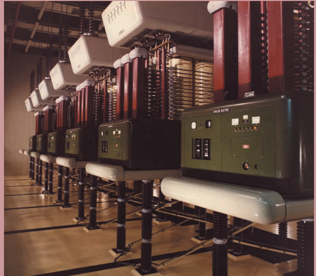
Nelson River HVDC Mercury Arc Valves
