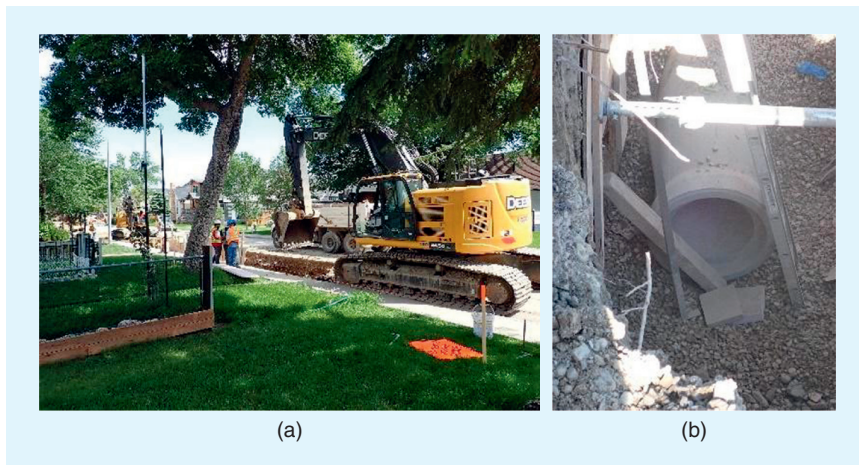
Figure 2: Photos of the construction of the Calgary public utility northwest inner city local and community drainage improvement project using the open cut method ( www.calgary.ca/planning/water/sunnyside-cdi.html ). (a) A crew digs the 5-m-deep trench along a residential street. (b) The trench has a concrete 0.6-m-diameter drainage conduit.
