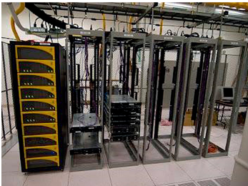
Figure 1: Common in data centres, 19-in. racks and cabinets are not ideal for shipboard use (Source: [2]; used with permission.)
